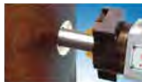
Strength weld removal prepares the surface for welding the new tube into place using the "Z Wart".
