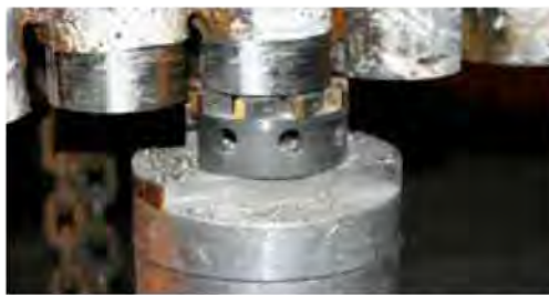
Overlay is removed from new and existing tubes and their ends are prepared for welding to new tubes.
