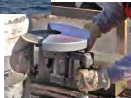
Scoring concrete pilings for height trimming. Concrete Cut-Off Blades are available in Diameters of up to 14”.
