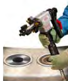
Bolt hole resurfacing is prepared using a standard Wart MILLHOG and cutter blades.
