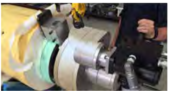
6" (152 mm) of polyethylene is removed from a steel pipe O.D. and beveled for welding spool pieces together.
